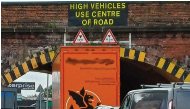
Harlaxton Road bridge, Grantham - struck 18 times in 2024/25. Perhaps not the most sensible signage! Photo: Network Rail
