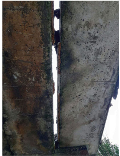
The bridge near Edderton, showing how far the beam was moved
